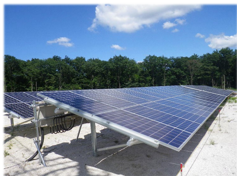
Kamonai Power Plant
